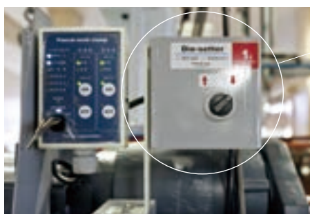
Die setter operation panel
