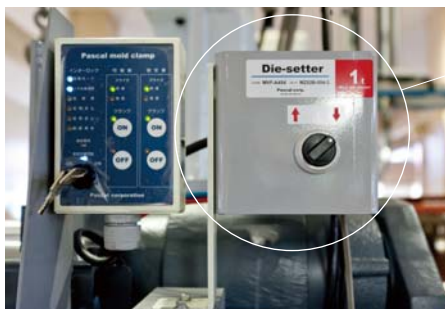
Die setter operation panel
