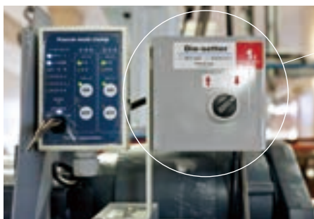
Die setter operation panel
