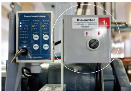
Die setter operation panel
